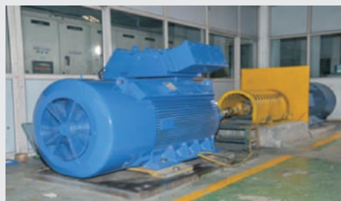
Large Motor Test Facility
