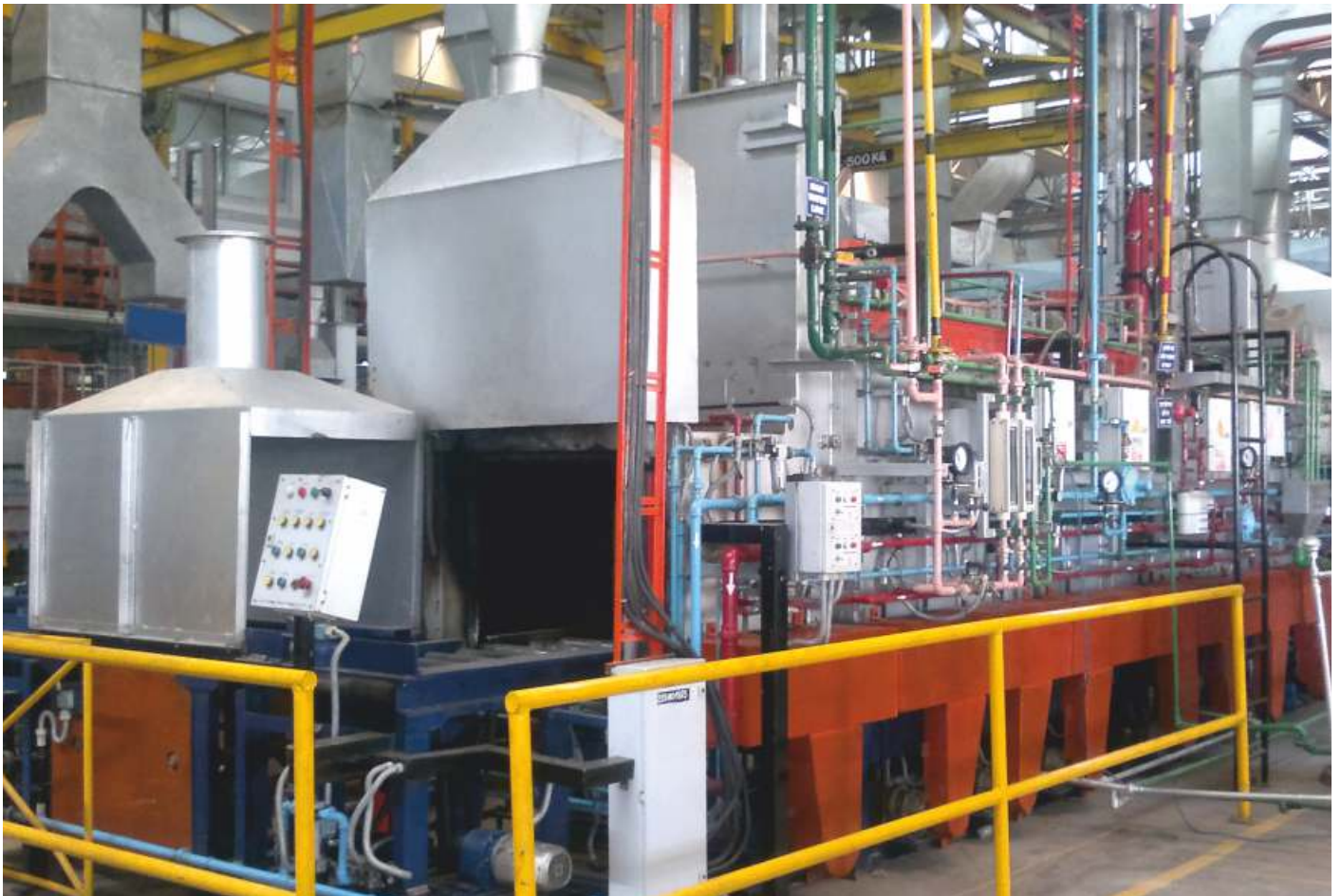
Continuous annealing furnaces (2 nos.) with capacity for processing 2000 kg/hour
